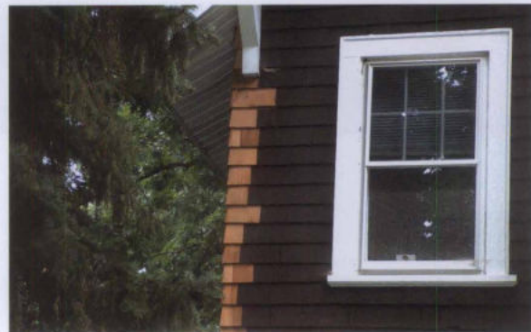
Figure 7. One of the advantages of wood shingles as a wall covering is that individual shingles that are damaged can easily be replaced. On this highly exposed corner, worn shingles have been selectively replaced to help safeguard against water damage. The new shingles will be stained to match the existing shingles.
