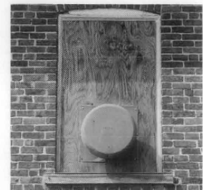
c. The exhaust fan has tamper-proof housing.
