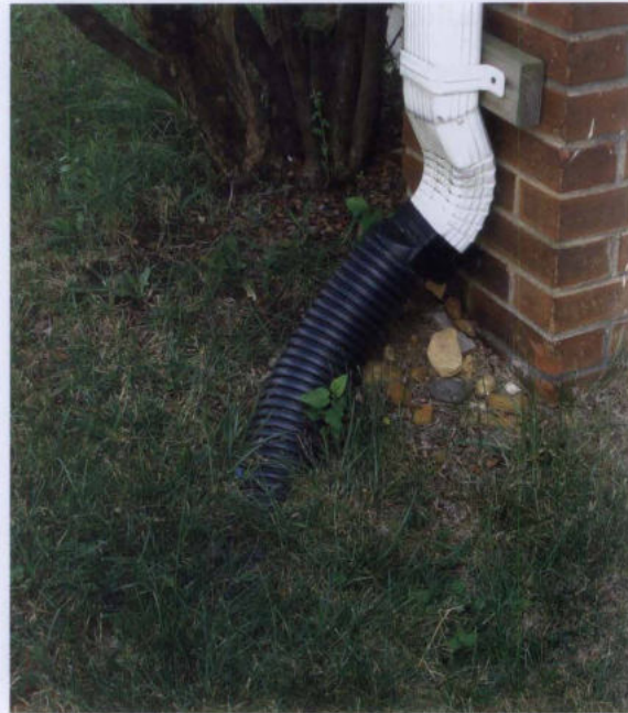
Figure 17. Extending downspouts at their base is one of the basic steps to reduce dampness in basements, crawl spaces and around foundations. Extensions should be buried, if possible, for aesthetics, ease of lawn care, and to avoid creating a tripping hazard. Photo: NPS files.
