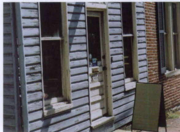
Figure 8. The paint on the siding of this south-facing wall needs to be scraped, sanded, primed and repainted. Postponing such work will lead to further paint failure, require greater preparatory costs, and could even result in the need to replace some siding. Photo: Charles Fisher.
