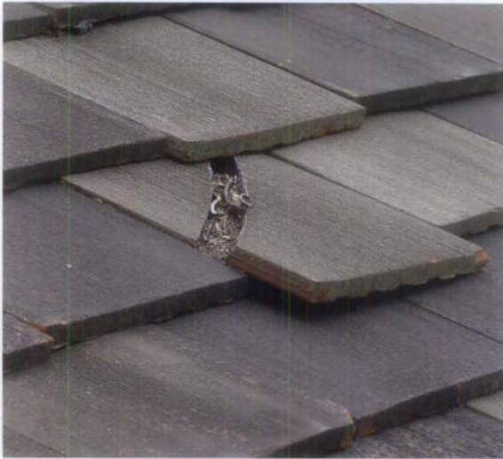
Figure 4. Damage to roofs often requires immediate attention. As a temporary measure, this damaged roof tile could be replaced with a brown aluminum sheet wedged between the existing tiles. Photo: Chad Randl.
