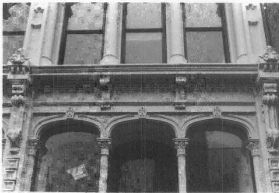
Figure 8. When the Grand Opera House in Wilmington, Delaware, was rehabilitated, missing cast-iron columns were cast of aluminum to match the original; in this particular case, because these columns do not carry great loads, aluminum proved to be successful substitute. Photo: John G. Waite
