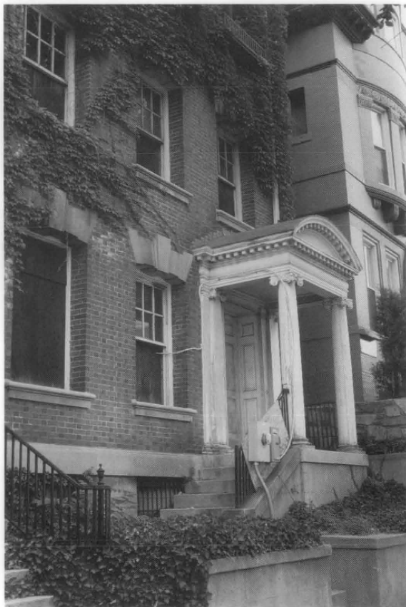
Figure 22. All systems except temporary electric have been shut off at this residence which has been mothballed over 20 years. An electric meter and 100 amp panel box have been set on a plywood panel at the front of the building. It is used for interior lighting and various alarm systems. The building, however, is showing signs of moisture problems with efflorescent stains on the masonry indicating the need for gutter maintenance and additional ventilation for the interior. The vegetation on the walls, although picturesque, traps moisture and is damaging to the masonry. Photo: H. Ward Jandl, NPS.
