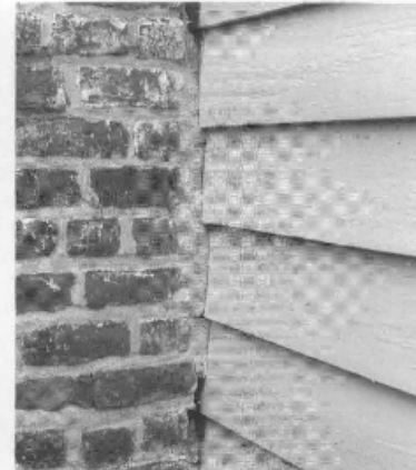
Figure 8. Appropriate mortar mixes should be used when masonry repairs are undertaken. In this case, a soft lime based mortar is used as an infill between the brick and wooden elements. When full repairs are made during the restoration phase, this soft mortar can easily be removed and missing bricks replaced.
