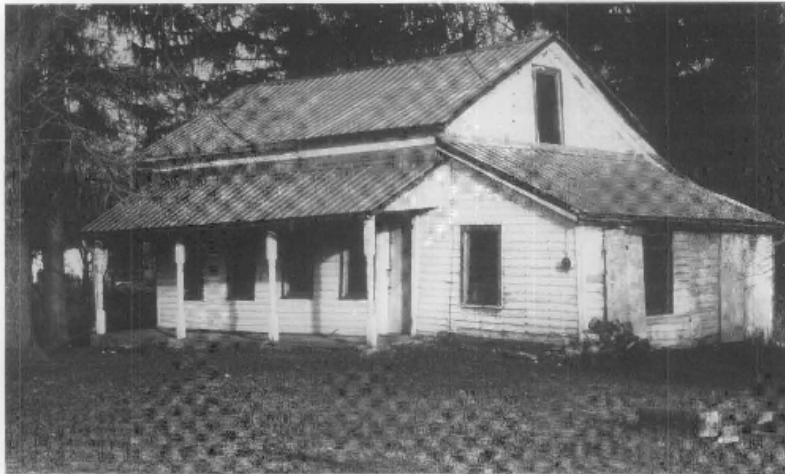
Figure 7. Non-historic materials are appropriate for mothballing projects when they are used to protect historic evidence remaining for future preservation. This lightweight aluminum channel frame and roofing covers the historic wooden shingle roof. Galvanized mesh panels secure the window openings from intrusion by raccoons and other unwanted guests. Photo: Williamsport Preservation Training Center, NPS.
