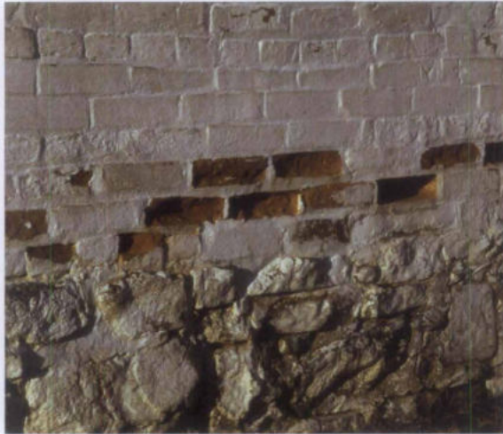
Figure 10. Repointing of masonry should usually be approached as repair rather than maintenance work in part because of the need for a skilled mason familiar with historic mortar. In this case, a moisture condition was not corrected and the use of a waterproof coating and off-the-shelf Portland cement mortar trapped water and resulted in further damage to these 19th century bricks. Photo: NPS files.
