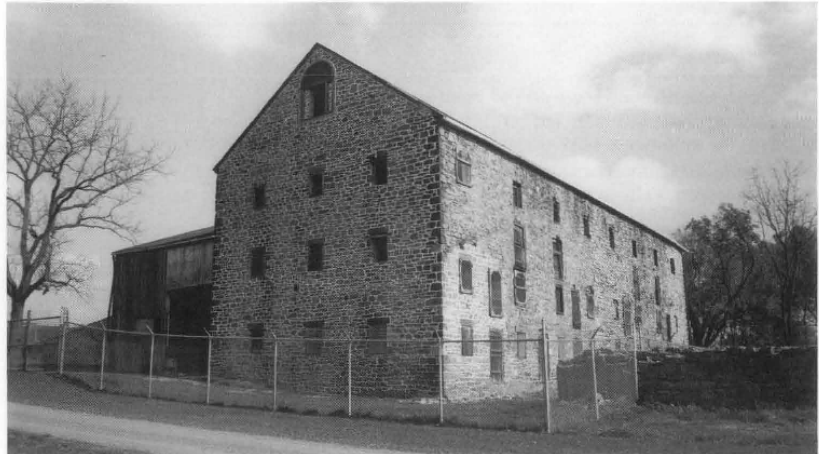
Figure 24. Once mothballed, a property must still be monitored and maintained. The openings in this historic barn have been modified with a combination of wood lowers and metal mesh panels which require little maintenance. The grounds are regularly mowed, even inside the chain link security fence. Photo: Williamsport Preservation Training Center, NPS.
