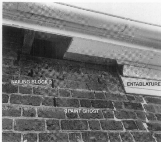
Figure A. Careful examination of the masonry reveals different periods of construction and repair through the composition and detailing of bricks and mortar. Depending upon location, open vertical joints may indicate the location of nailing blocks for decorative trim or weeps for drainage. These open joints at the building's cornice show evidence of an earlier wooden entablature extending down two courses below the present trim. The paint ghosts below the lowest blocks confirms the entablature's existence and provides clues to its size and finish.
