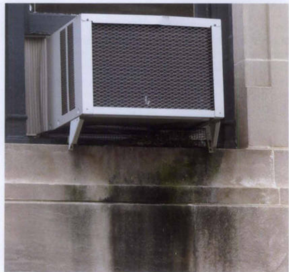
Figure 13. Window air conditioning units can cause damage to surfaces below when condensation drips in an uncontrolled manner. Drip extension tubes can sometimes be added to direct the discharge.
