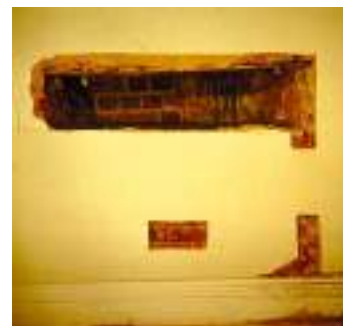
Exploratory testing was used to verify the location of an abandoned fireplace. Plaster and brick were carefully documented and removed to determine the fireplace's type, size, and location. Photo: Travis C. McDonald, Jr.
