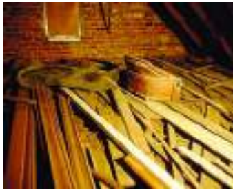
Discarded items are routinely stored within attics, then forgotten only to be discovered during a later investigation. Seemingly worthless debris may help answer many questions. Photo: Travis C. McDonald, Jr.
