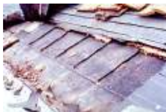
In many cases, new materials or coverings are placed directly over existing exterior features, preserving the original materials underneath. Here, the removal of a modern shingle roof and its underlayment revealed an historic standing seam metal roof. Photo: Courtesy, Phillips and Opperman, P.A.
