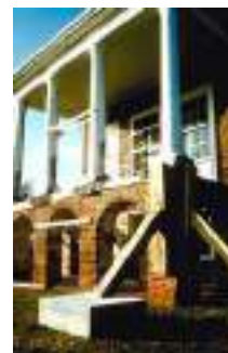
Investigation frequently identifies urgent needs of stabilization. Supplemental support, such as temporary shoring, may be required to prevent collapse. Photo: Travis C. McDonald, Jr.
