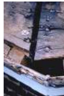
Analyzing the nail technology can help establish the period of construction and provide other important information. Photo: Travis C. McDonald, Jr.
