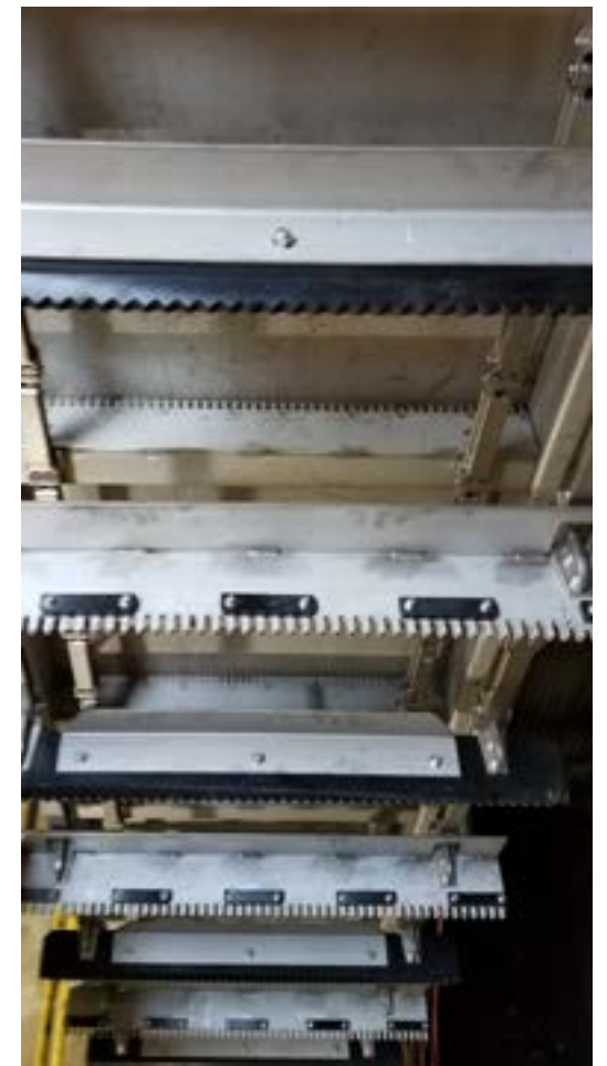
(Above: newly installed Bar Rakes which prevent rags and larger debris from destroying the pumps and equipment)
